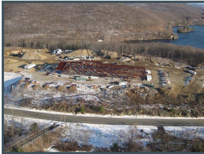
Akima's equipment maintenance group at West Point is scheduled to take occupancy at the new transportation and maintenance facility by June 2010. The operations and project management group will follow by September 2010.
