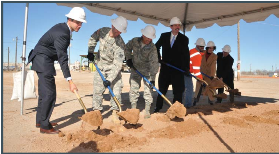
On December 15, 2009 the U.S. Air Force broke ground on a $10 million fuel storage facility that is expected to be completed by December 2010 at Kirtland AFB.
